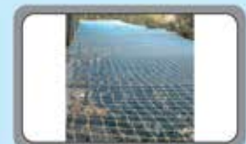
Under Construction Safety net
