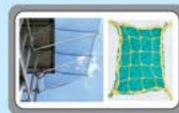
Under Construction Safety Net
