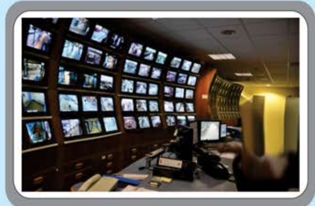
CCTV Control Room
