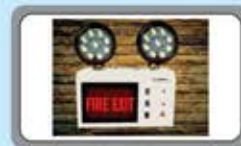
Emergency Exit Signages
