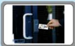
Access Control System
