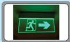
Emergency Exit Light
