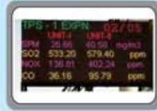
Pollution Control Data Display Board
