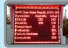
Pollution Control Data Display Board
